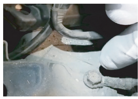
Check For Corrosion at The Connection Under The Battery Tray of Toyota Vehicles
